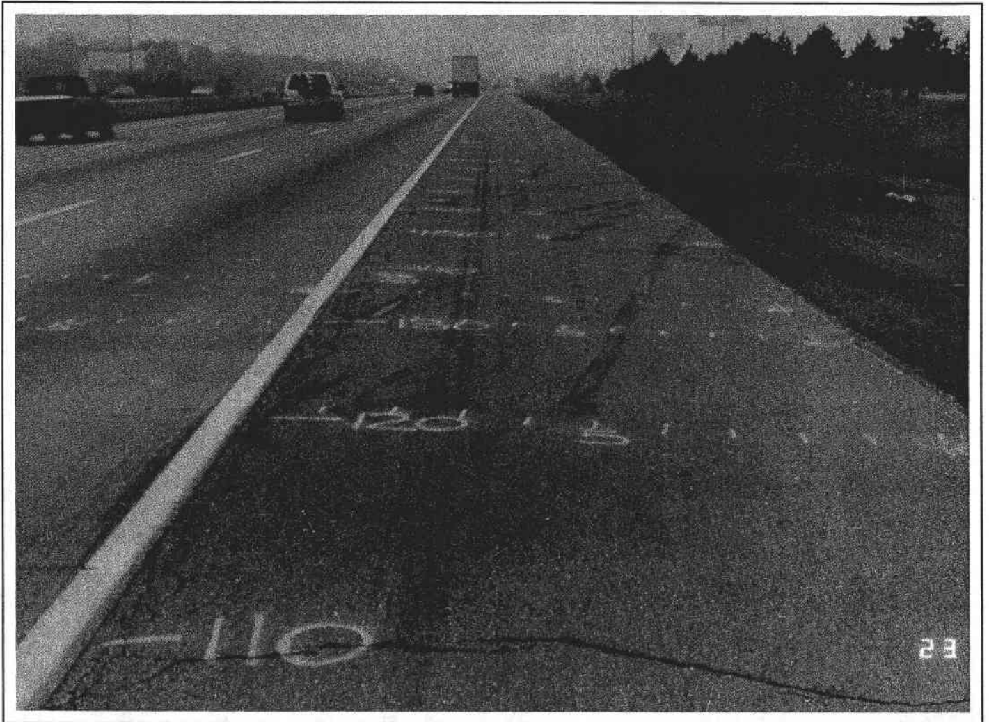
Figure 12 - Detailed grid placed on an interstate shoulder to document a complex array of skid and gouge marks.
